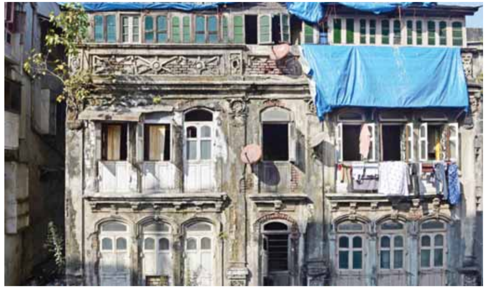
A dilapidated building in the Bhandi Bazaar area of Mumbai that is being redeveloped under the Cluster Development Act 2009 by the Saifee Burhani Upliftment Trust.
