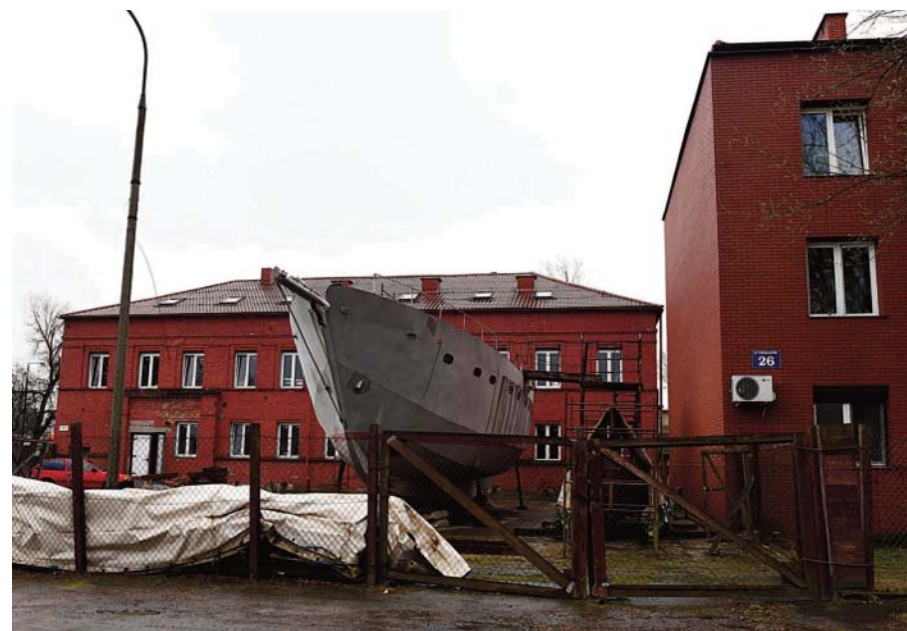
WARSAW: A steel schooner called 'Father Boguslaw' is under construction at the courtyard of a homeless shelter run by Catholic Fathers in Warsaw. —AFP
