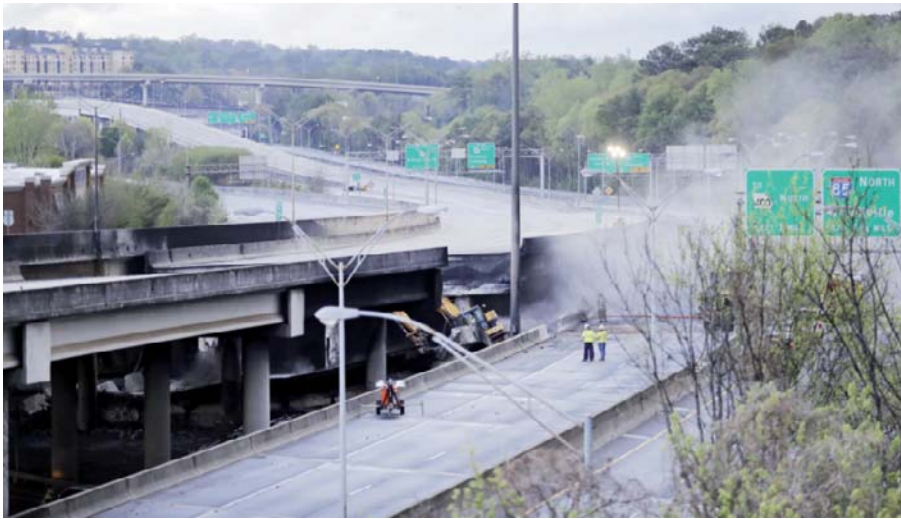
ATLANTA: Crews work on a section of an overpass that collapsed from a large fire on Interstate 85 in Atlanta. — AP
