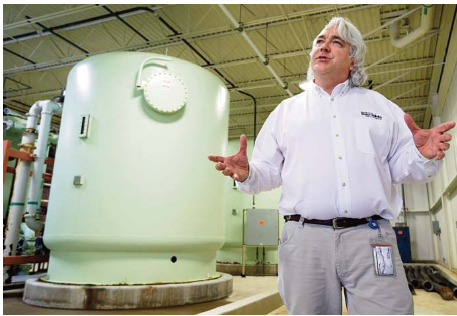
DES MOINES: Des Moines Water Works CEO Bill Stowe stands in the Nitrate Removal Facility at the Water Works treatment plant in Des Moines, Iowa. For years the utility that supplies drinking water to the state's capital city has spent millions of dollars to rid its water supply of pollutants that run off farm fields. —AP
