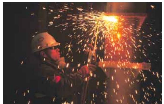
QINGDAO, China: Sparks fly as a welder works in a subsidiary of China Offshore Oil Engineering Co Ltd in eastern China's Shandong province yesterday. — AP
