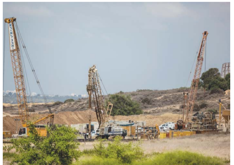
In this Thursday, Sept. 8, 2016 file photo, heavy machinery works on a massive underground barrier on the Israeli side of the border with Gaza. —AP
