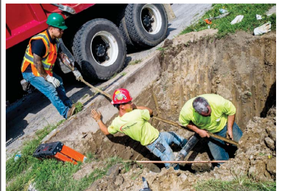
FLINT, Michigan: In this Aug 31, 2016 photo, crews break ground and work to remove and replace lead-tainted pipes from three homes. — AP
