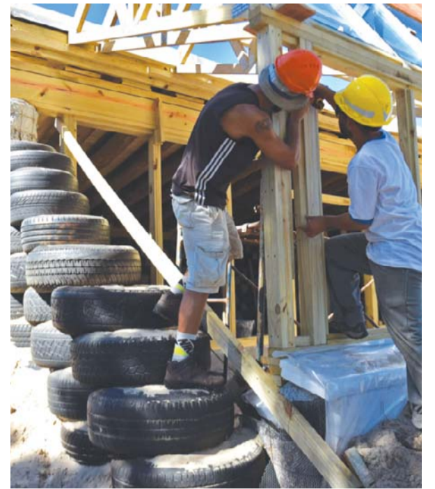
JAUREGUIBERRY, Uruguay: Trainees work during the construction of an auto-sustainable elementary school in Jaureguiberry.
