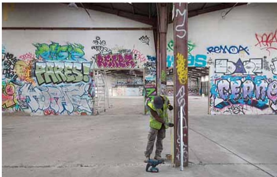
PARIS: This file photo taken on August 30, 2016 shows a worker on the construction site of a future migrant camp. —AFP
