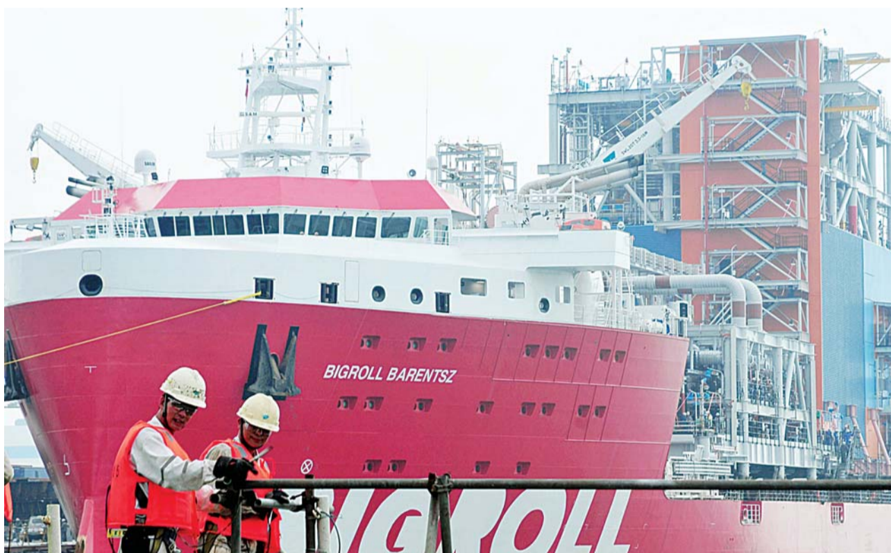
QINGDAO: Chinese workers install scaffolding at an offshore oil engineering platform in Qingdao, east China's Shandong province yesterday. —AFP
