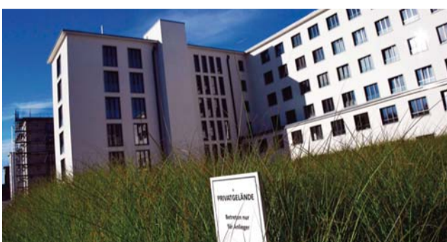
A construction site of luxury apartments as part of transformation of the heritage-protected Prora Complex.
