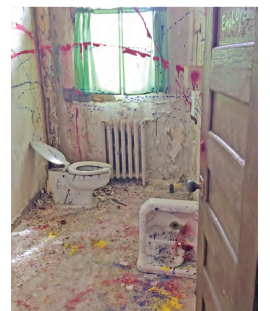
A vandalized bathroom is shown inside an abandoned building at the former Mansfield Training School in Mansfield, Conn.
