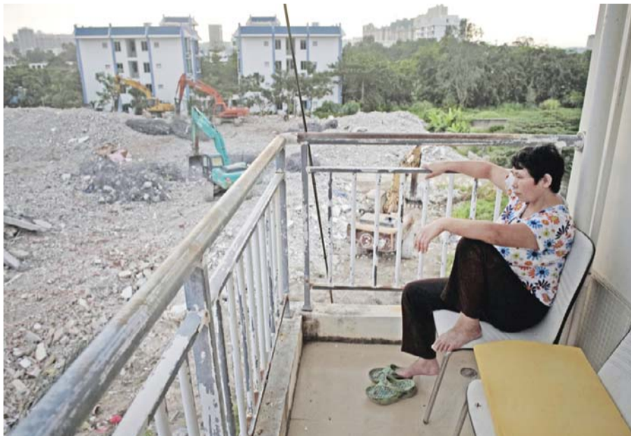
BEIJING: A woman sits on her balcony as she watches bulldozers clearing the rubble of demolished buildings to clear the ground for a new property development project in Sanya. — AFP
