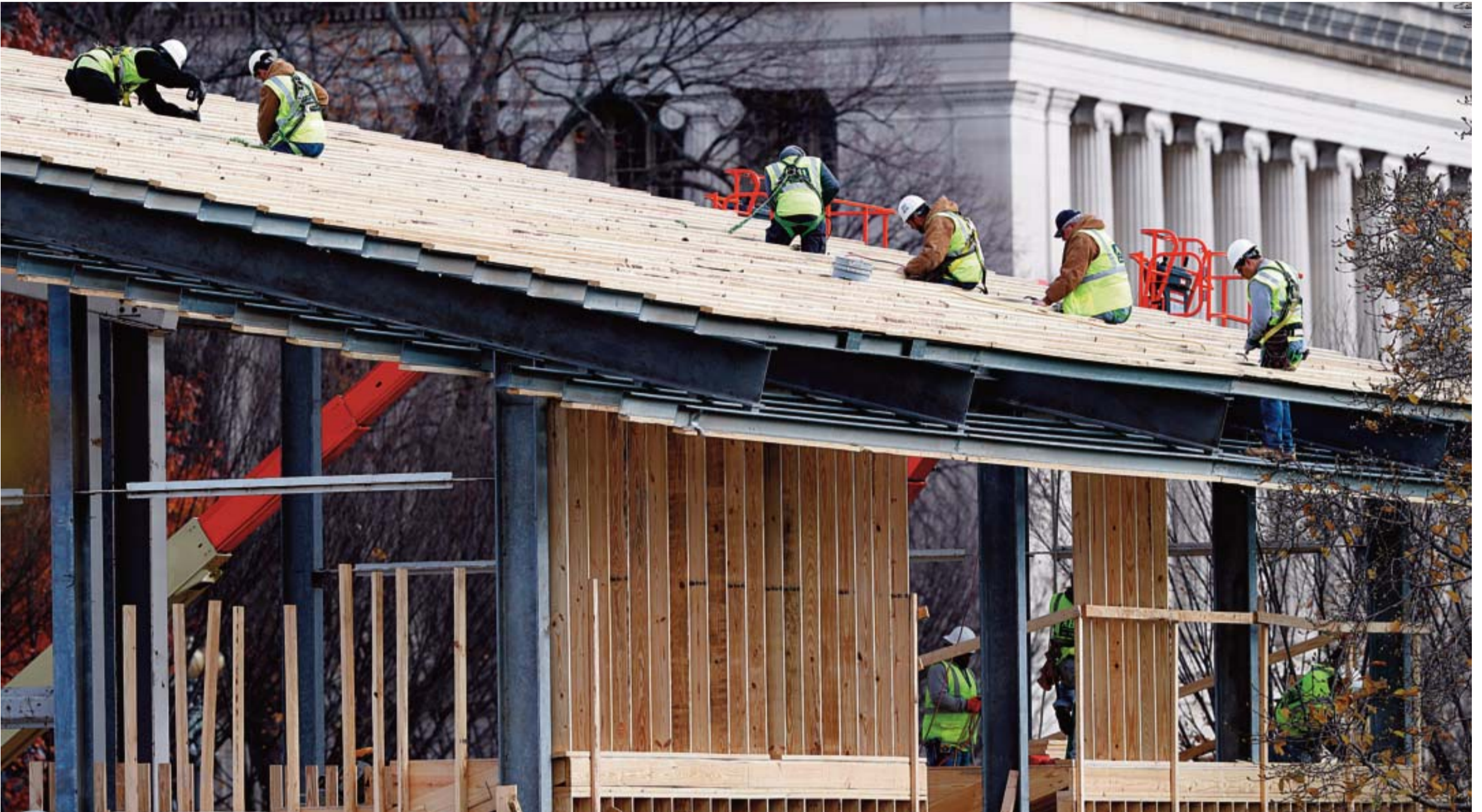
WASHINGTON: Construction continues on the presidential reviewing stand on Pennsylvania Avenue in front of the White House, Saturday, Nov 26, 2016. —AP
