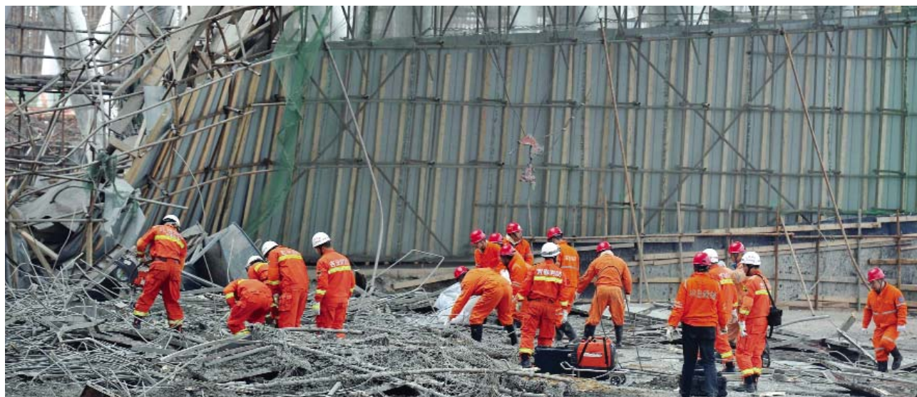
FENGCHENG, China: Workers search for survivors in the debris of a collapsed platform in a cooling tower at a power station at Fengcheng, in China's Jiangxi province yesterday.—AFP
