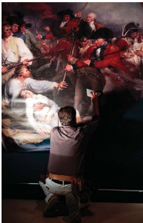
In this photo, under a spotlight, Gary Davis, hangs a mural depicting the Battle of Bunker Hill as construction continues at the Museum of the American Revolution in Philadelphia.
