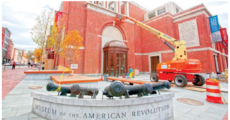
In this photo, construction continues on the exterior at the Museum of the American Revolution in Philadelphia.
