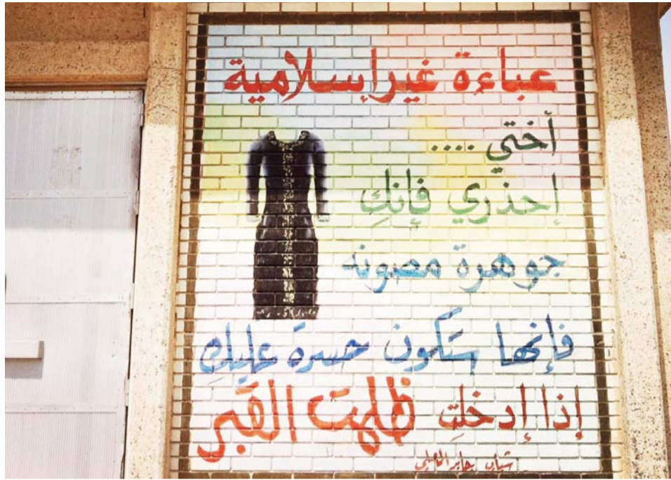
'This is an unislamic abay', be careful, you're a preserved diamond, and it will be a huge regret when you enter into the darkness of grave'. These comments are painted on electric substations in some residential areas of Kuwait. — Photos by Athoob Al-Shuaibi
