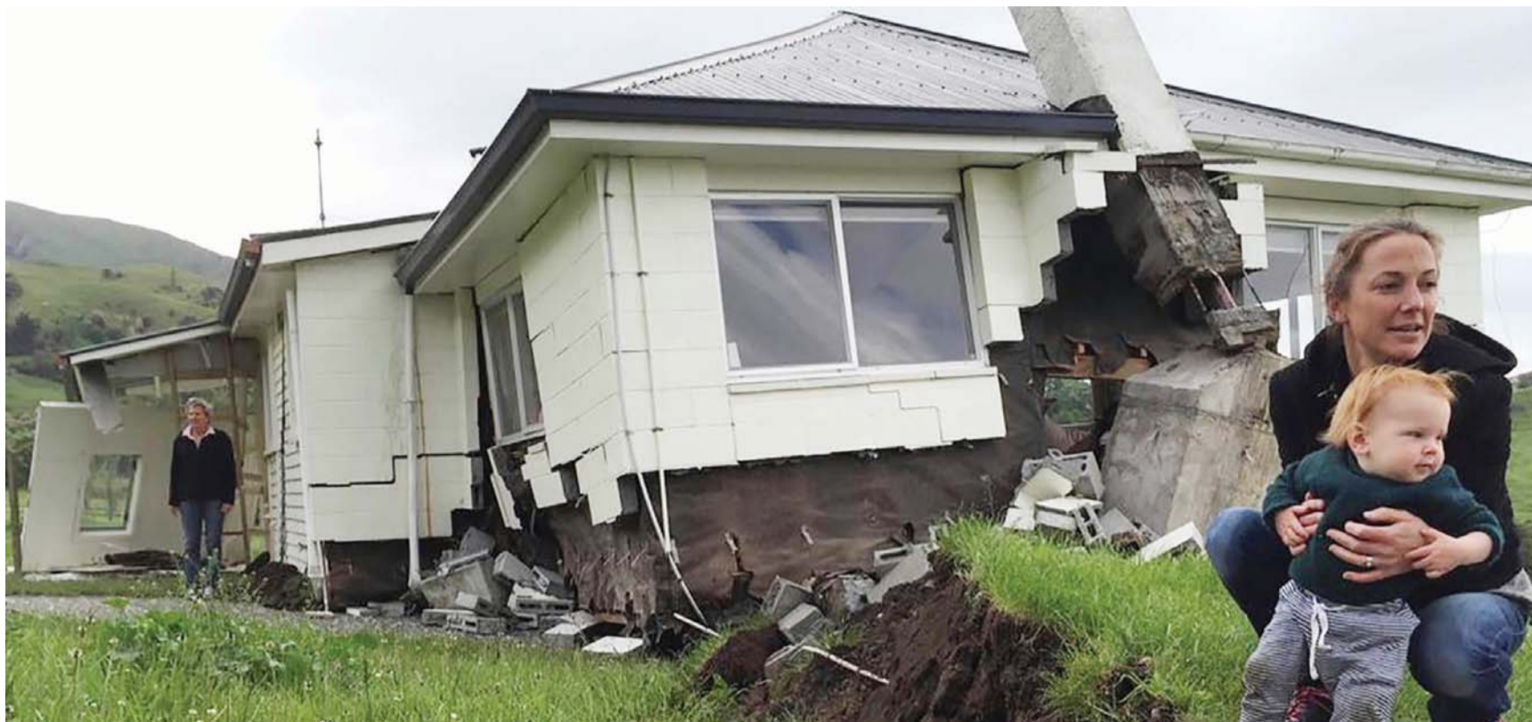
BLUFF STATION, New Zealand: A woman and child are seen in front of a house damaged by an earthquake as it sits on the fault line near Kaikoura on the South Islands east coast. —AFP
