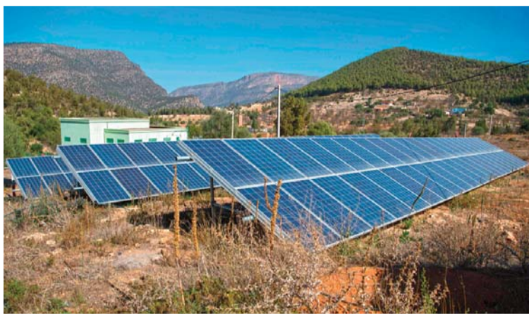
TAFOUGHALT, Morocco: A general view shows solar panels that are connected to a generator which feeds a pump extracting water from underground in Tafoughalt, a little village deep in the mountains of Morocco's eastern Berkane province. — AFP
