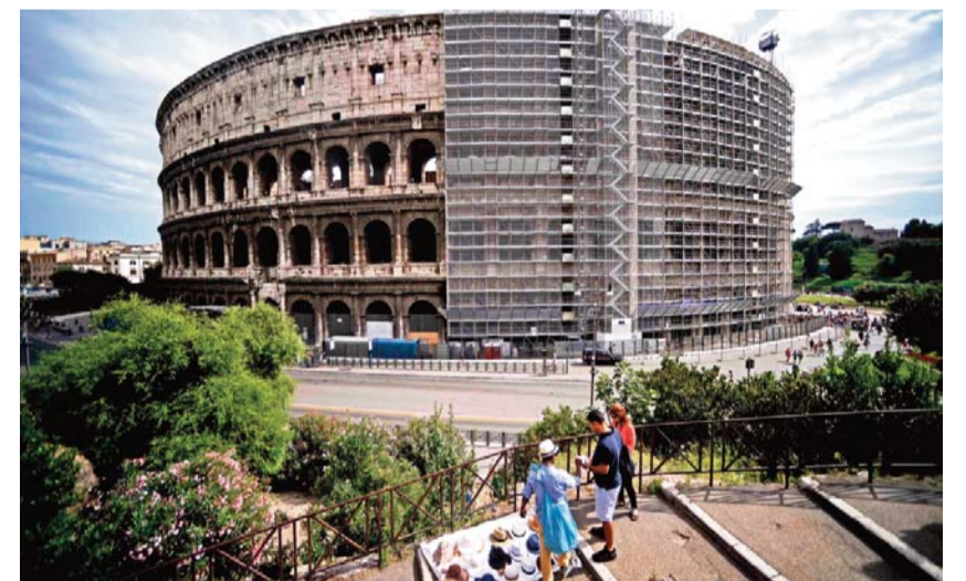
A general view shows the scaffoldings of the Colosseum (Coliseum) during the restoration funded by Italian brand 'Tod's' in Rome. — AFP photos
