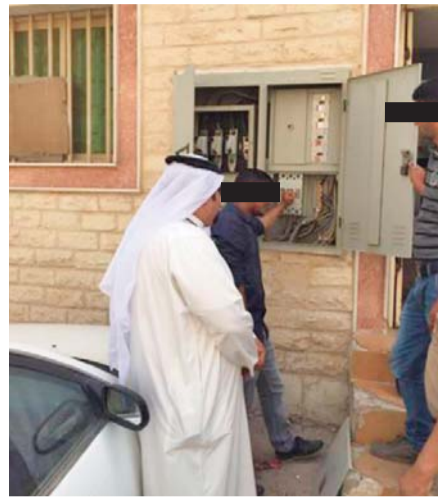
A Kuwait Municipality inspector oversees the process of disconnecting power from violating buildings.
