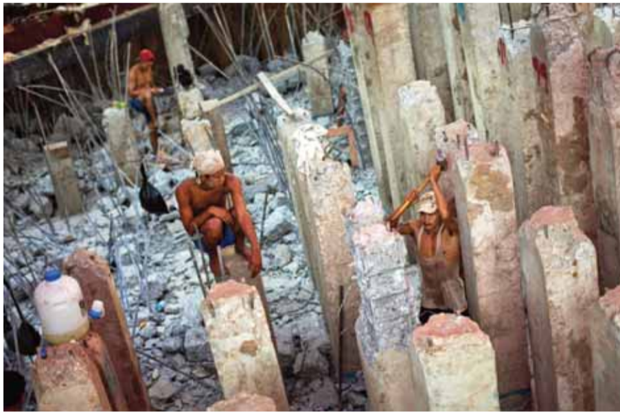
YANGON: Myanmar construction workers partially demolish a foundation of a building under construction. — AFP
