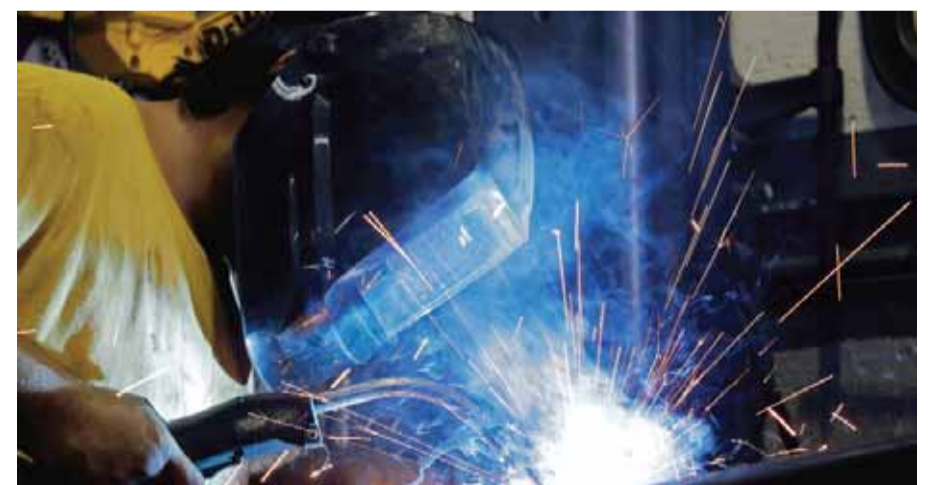
HIALEAH, Florida: Welder Gabriel Gonzalez welds a support beam at a local welding shop. — AP
