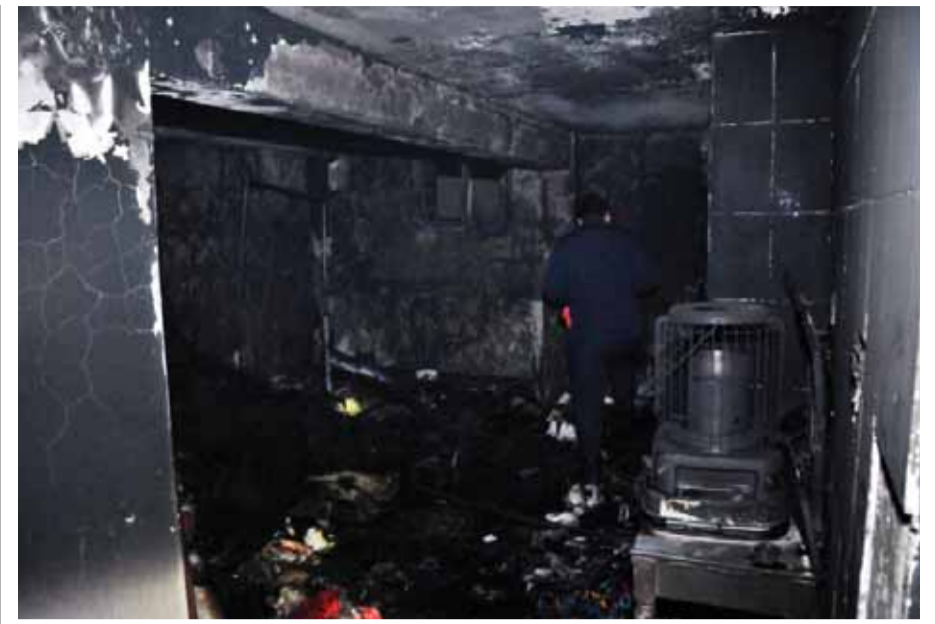
KUWAIT: A firefighter inspects damage after a blaze was put out inside an apartment in Saad Al-Abdullah yesterday.
