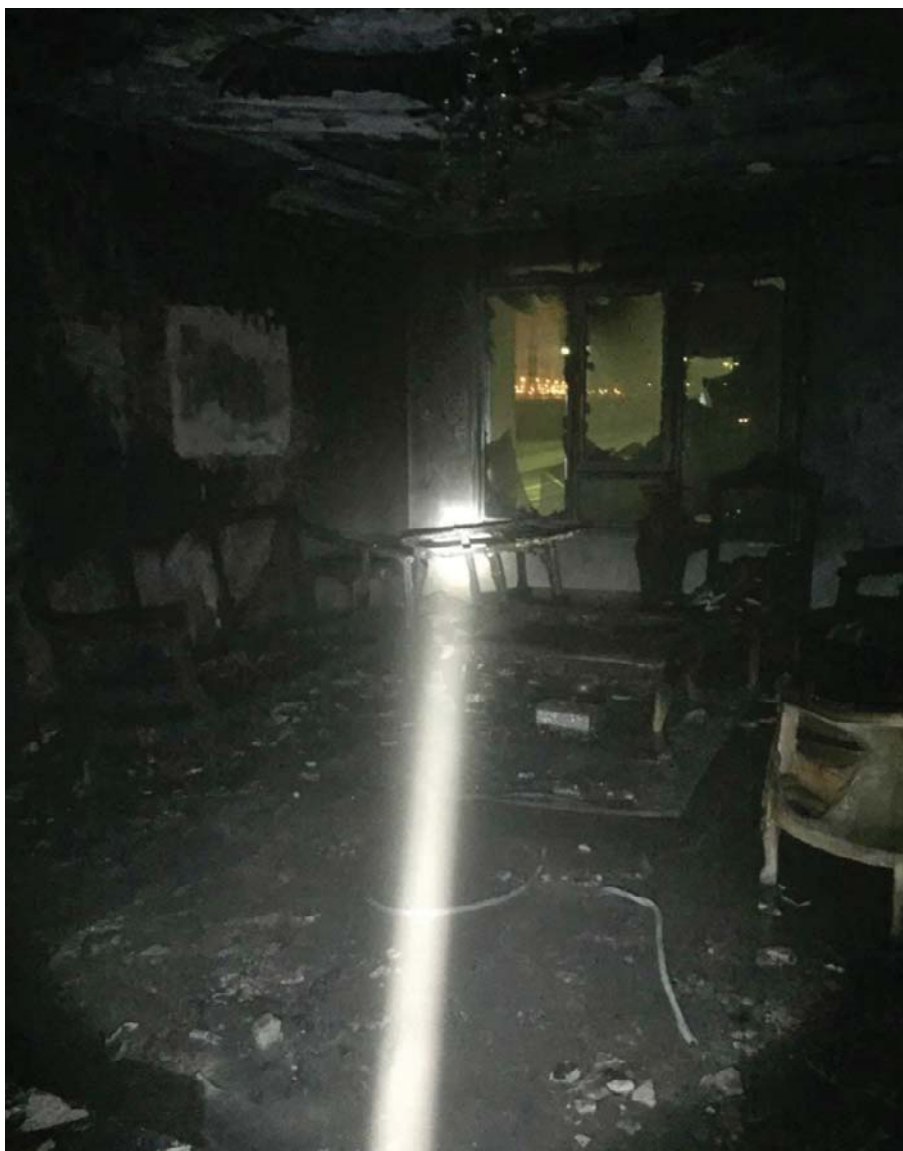
KUWAIT: Firefighters inspect the scene after tackling a blaze inside in Abdullah Mubarak house.
