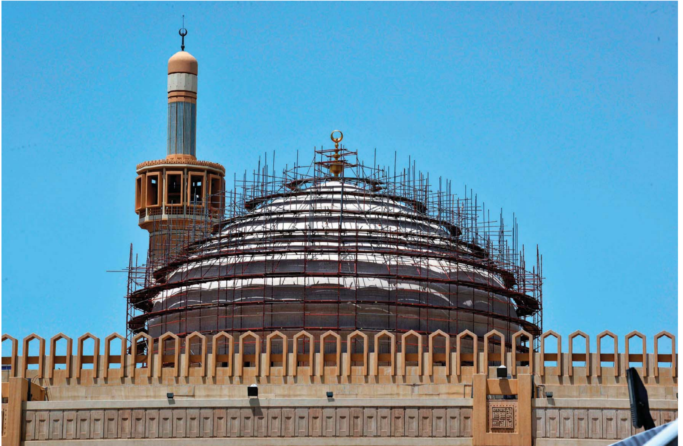
KUWAIT: Restoration works at the Grand Mosque's dome, which are set to finish before the beginning of the holy month of Ramadan. — KUNA
