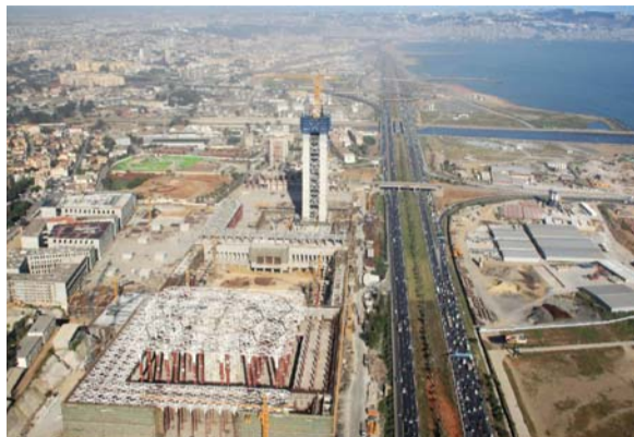
An aerial view taken on April 26, 2016, from a police helicopter above Algiers shows the construction site of the third largest mosque in the area and the largest in Africa. — AFP
