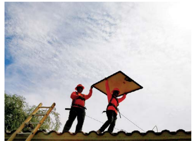
GOOD YEAR: Electricians install solar panels on a roof for Arizona Public Service company in Goodyear, Ariz. Wind turbines and solar panels accounted for more than two-thirds of all new electric generation capacity added to the nation's grid in 2015, according to a recent analysis by the US Department of Energy. The remaining third was largely new power plants fueled by natural gas, which has become cheap and plentiful as a result of hydraulic fracturing. — AP
