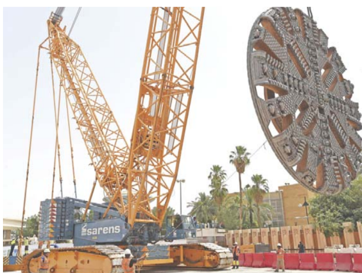
RIYADH: Foreign engineers work yesterday at a construction site of a section of the capital's $22.5 billion metro system. — AFP
