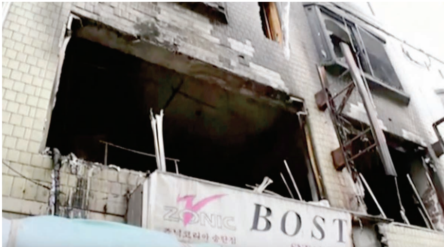
PYEONGTAEK, SOUTH KOREA: A building is burned after a fire where residents, including US servicemen, used a blanket to catch a woman and her three children as they jumped to safety. — AP
