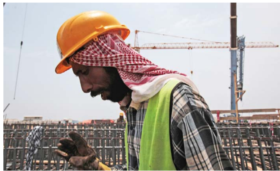
JEDDAH: In this May 8, 2014 file photo, a man works on construction of the Kingdom Tower, a planned 252-storey building which aims to become the world's tallest skyscraper when complete. — AP
