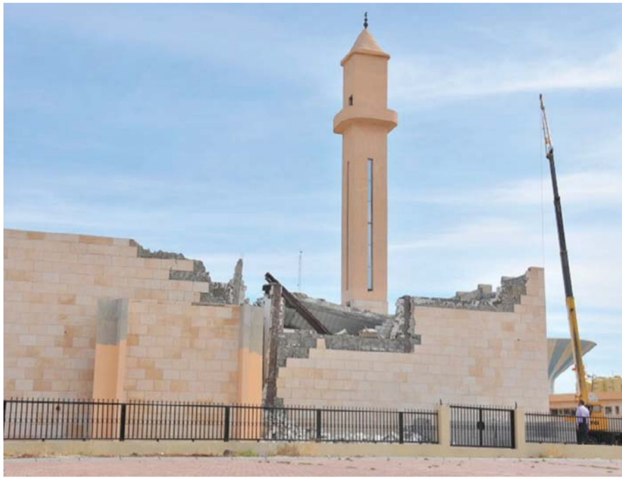
KUWAIT: Damages are seen at a mosque under construction in Qairawan after the roof collapsed yesterday, leaving four workers injured.
