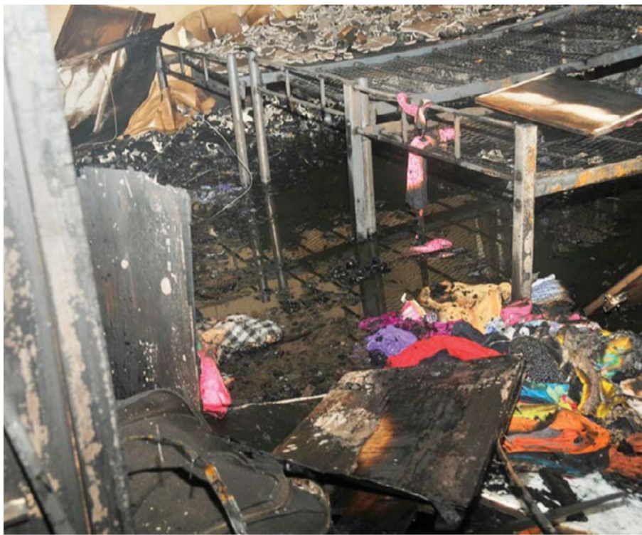
The scene at a house's basement in Sabah Al-Nasser after fighters tackled a blaze there.
