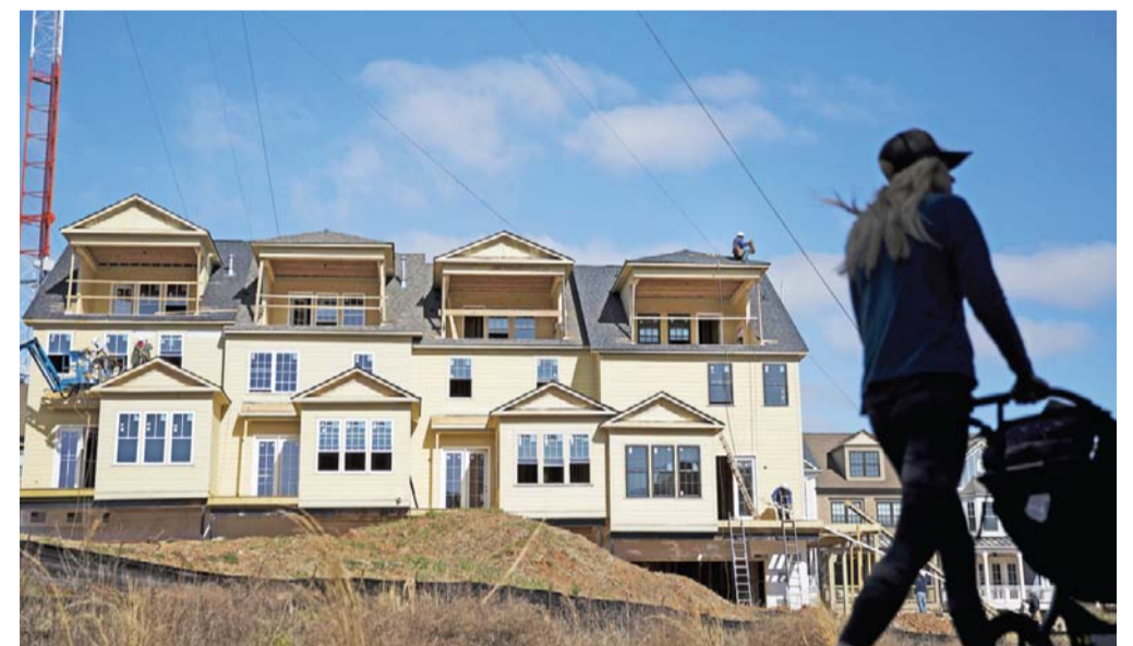
ATLANTA: Town homes stand under construction as a pedestrian walks along the BeltLine in Atlanta. Standard & Poor's/Case-Shiller yesterday issued its 20-city home price index for January. — AP
