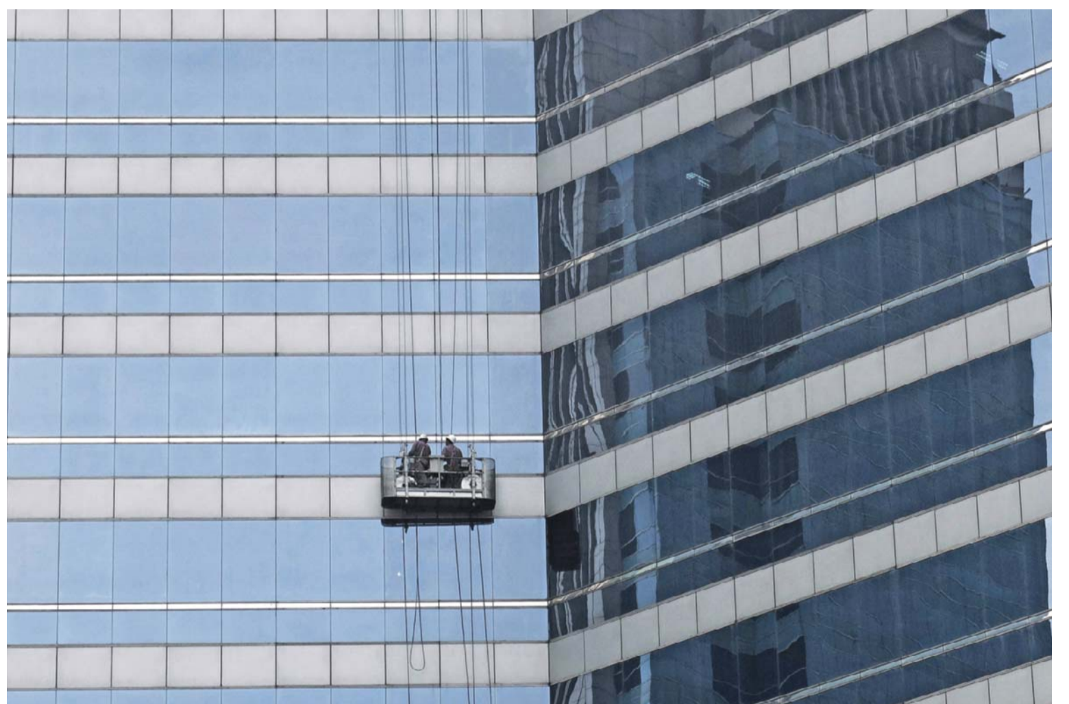
JAKARTA: Workers clean windows on one of the skyscrapers in Jakarta yesterday. Indonesia's central bank cut its key interest rate for the third straight month, encouraged by lower inflation and a stronger currency in Southeast Asia's top economy. —AFP
