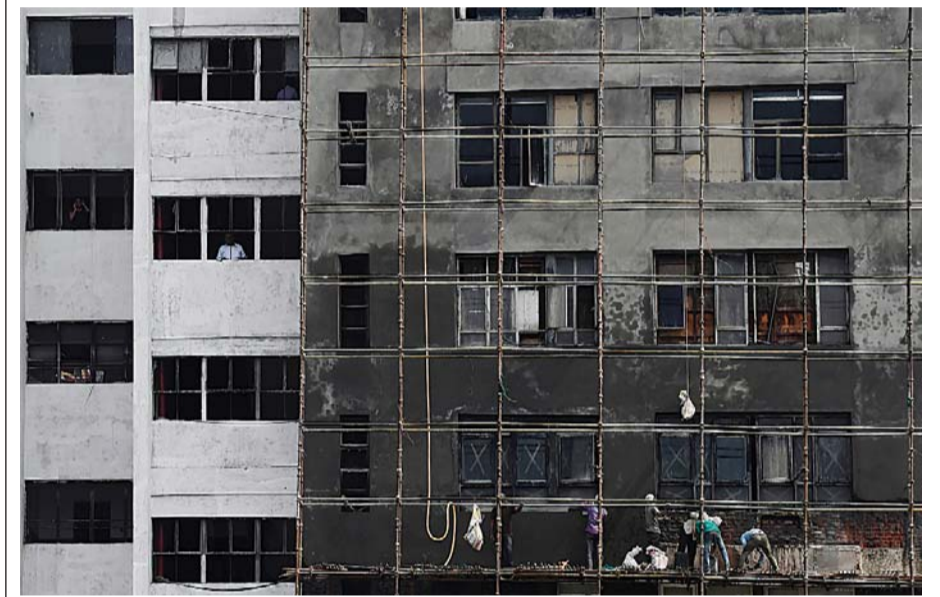
NEW DELHI: Indian laborers renovate the outer facade of a building in a business district of New Delhi yesterday. India is now the world's fastest-growing major economy, but two years of drought and a failure to create jobs for a burgeoning young population has left millions of rural residents struggling, and led to deadly protests in recent weeks.—AFP
