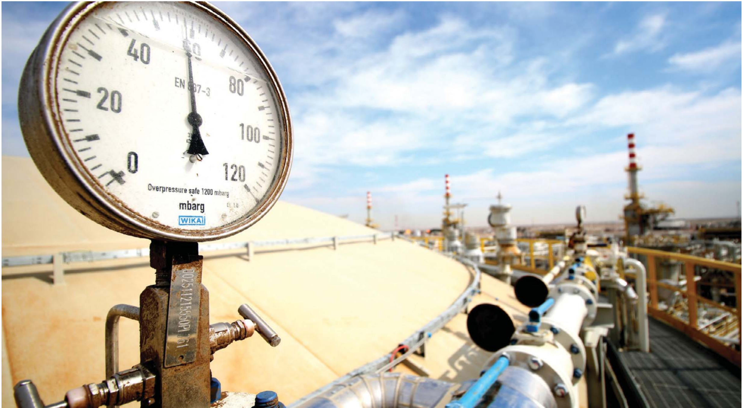
BASRA: A general view shows pipelines in the newly opened section of the oil refinery of Zubair, southwest of Basra in southern Iraq. Iraq's oil exports and revenue dipped in February compared with the previous month as low global crude prices offered Baghdad no financial respite. — AFP
