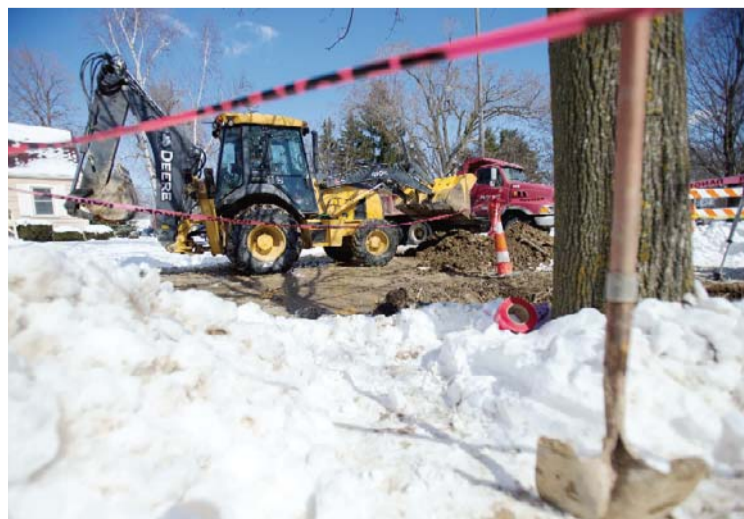
MICHIGAN: Workers move dirt in front of a home in Flint, Michigan as they replace the old lead pipe with a new safer copper pipe. — AFP
