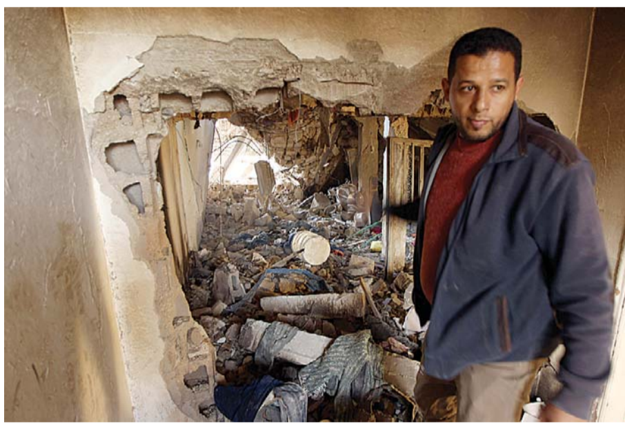
LAITHI: A Libyan man inspects the damage in a destroyed building in Laithi district, a central area that was recently re-seized by forces loyal to Libya's internationally recognized government in the eastern coastal city of Benghazi. —AFP
