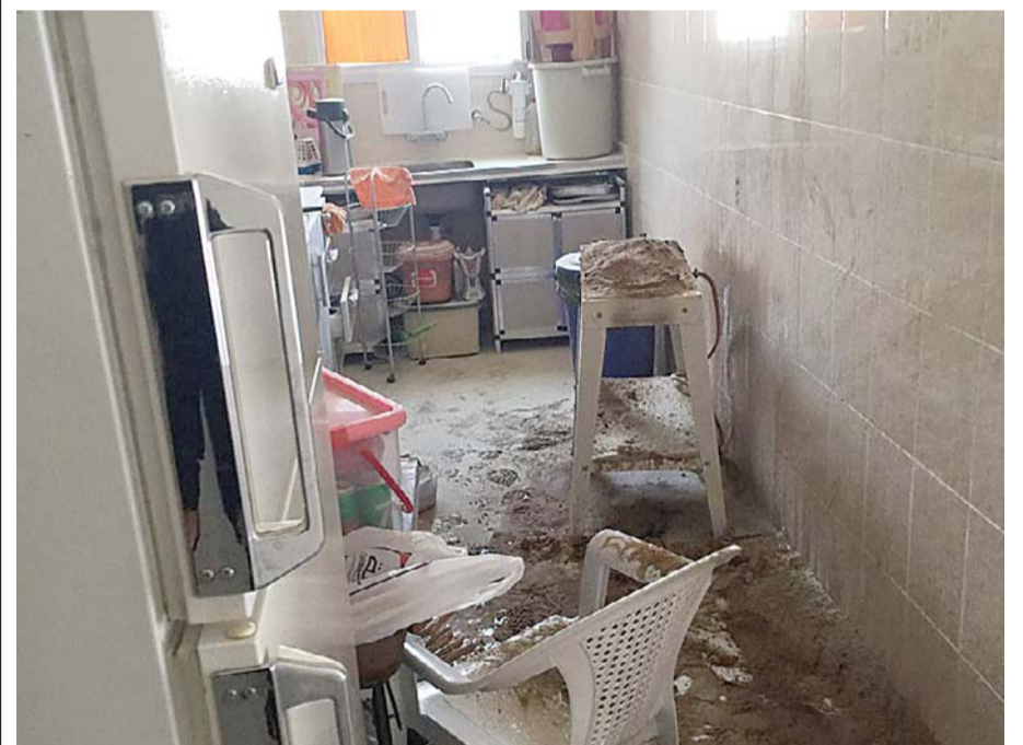
The scene after a fire was put out inside a Wafra farm's kitchen.
