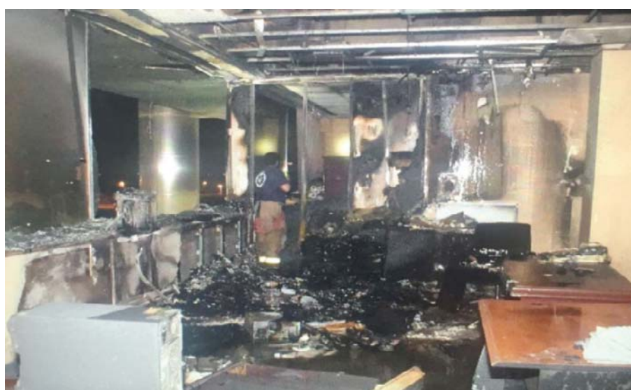
KUWAIT: A fire broke out at Nawaf Al-Ahmad building and resulted in minor material damage, the Ministry of Interior said Saturday night. The firefighters responded promptly to the fire and managed to subdue it timely, the Ministry's Security Media Department said in a press release.— KUNA
