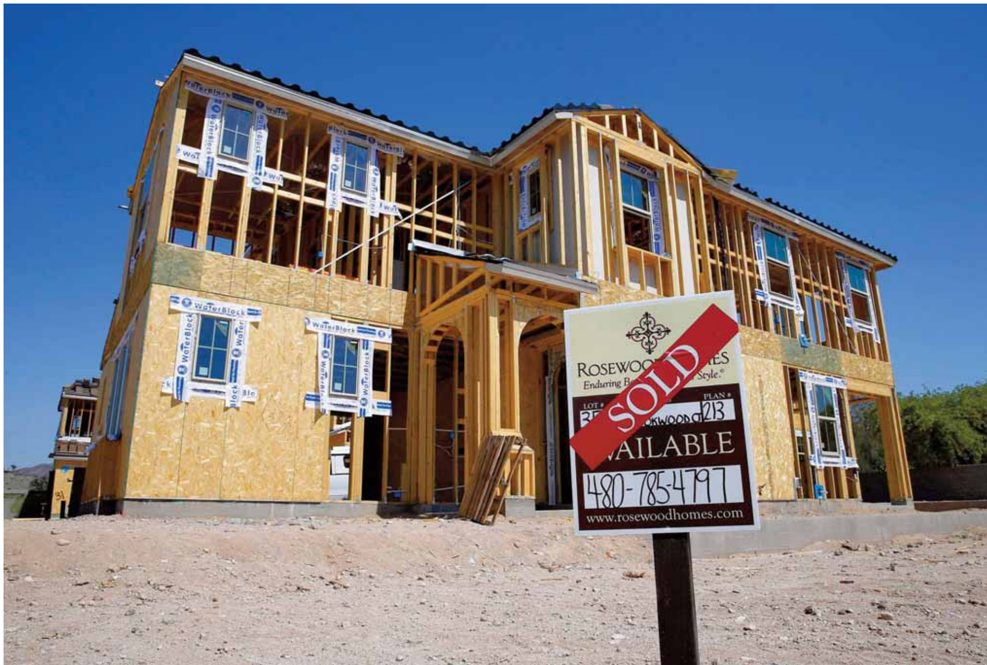
PHOENIX: A new home under construction in Phoenix. The Commerce Department Reported yesterday on US home construction in May. — AP
