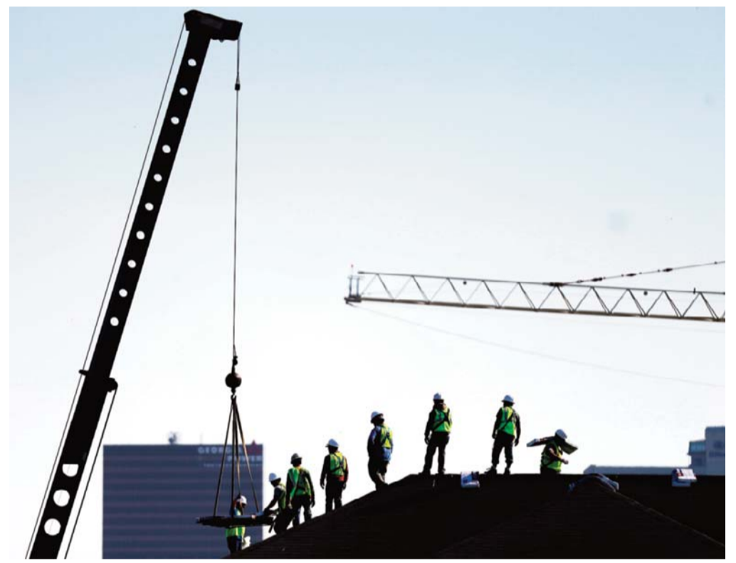
ATLANTA: Construction workers unload supplies off a hoisted pallet on a rooftop in Atlanta. Yesterday, the Labor Department issues revised data on productivity in the first quarter. — AP
