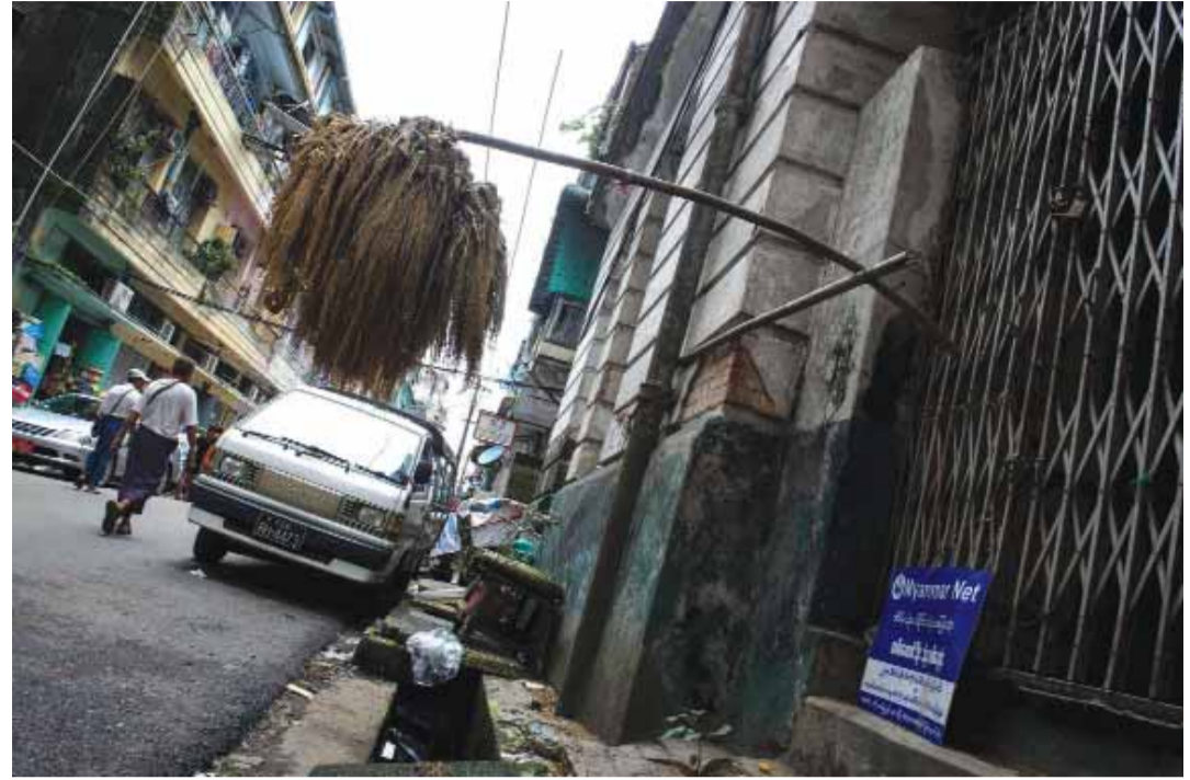
YANGON: A rice straw bundle for feeding birds hangs from the door of the abandoned colonial building that was the former headquarters of Burma Oil during the British rule. — AFP
