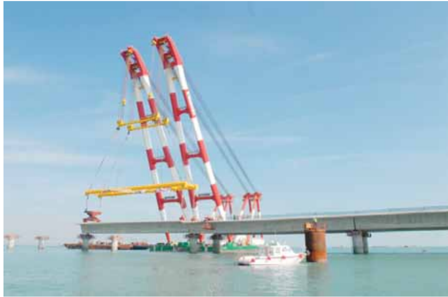
KUWAIT: Ongoing construction works at the Sheikh Jaber Al-Ahmad Causeway project. —KUNA
