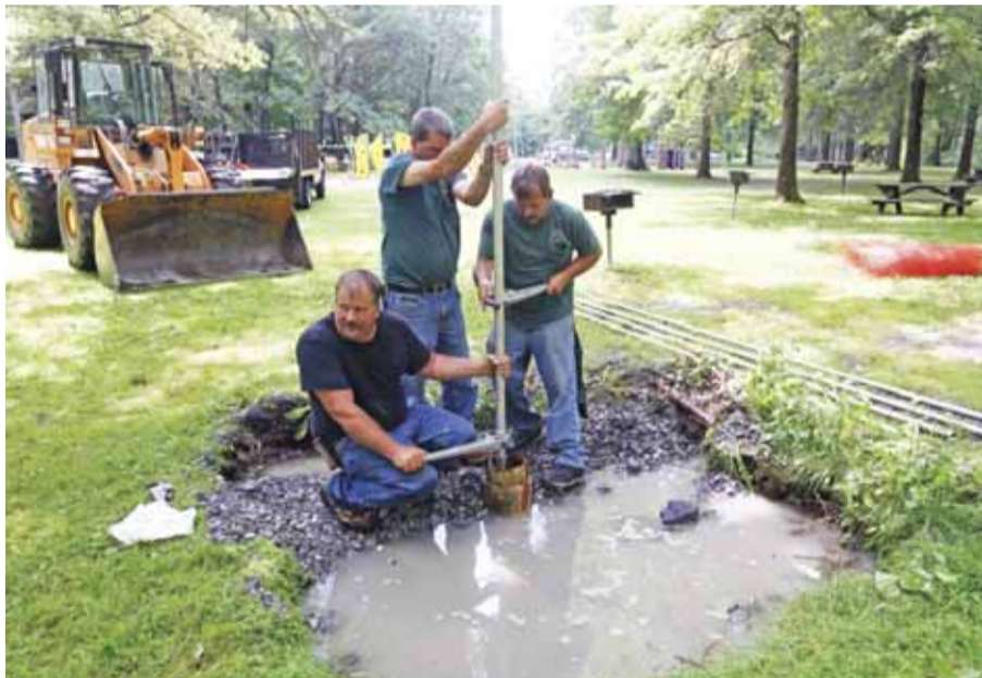
NEW YORK: In this photo, state parks workers Mark Holmes, Jay Downing and Rod MacDuff connect pipes on Shonts Well # 3 that is being in restored at Saratoga Spa State Park in Saratoga Springs, New York. — AP
