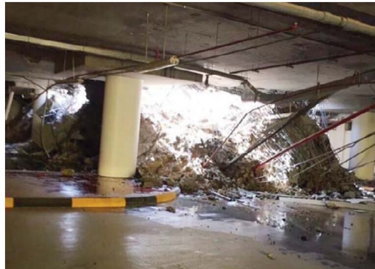
KUWAIT: This handout photo shows debris at the site of the collapse reported yesterday at a college in Ardhiya.
