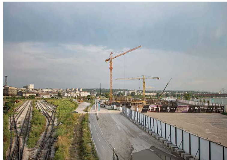
BELGRADE: Photo shows the construction site of the Belgrade waterfront project. Authorities say the $3 billion (2.7-billion-euro) project, led by Abu Dhabi-based developer Eagle Hills, will generate thousands of jobs and much-needed investment, as well as revamping rundown parts of the banks of the River Danube for public use.—AFP
