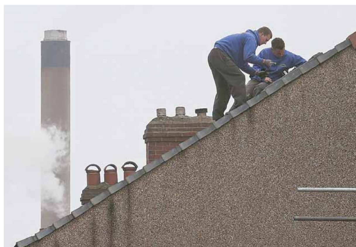
PORT TALBOT, UK: Builders working on the roof of a residential property near the Tata Steel steel plant at Port Talbot, south Wales. —AFP
