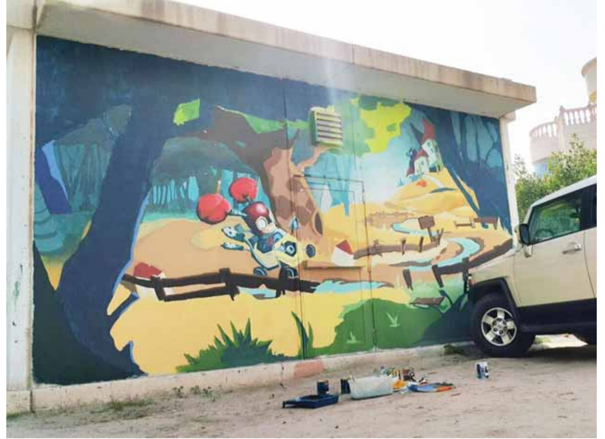
Power transformer (after).
