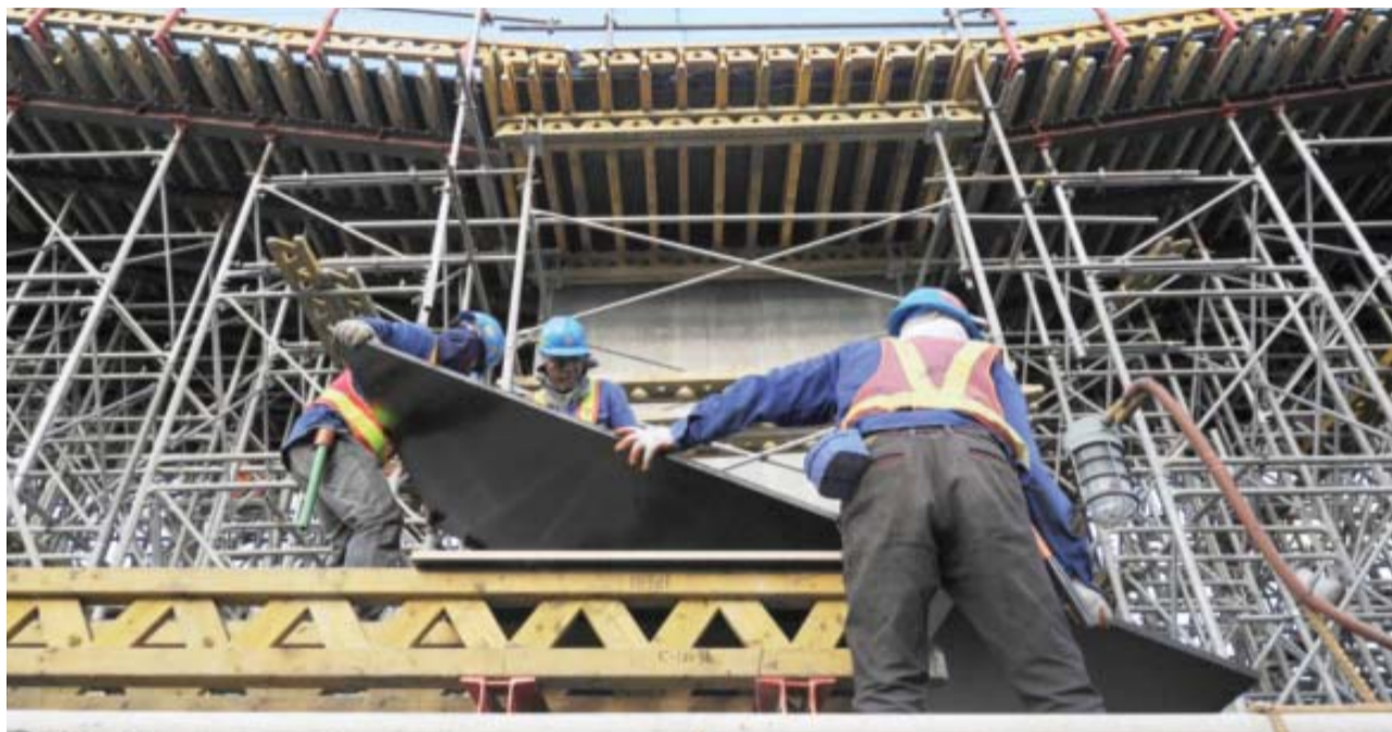
MANILA: Construction personnel work beside scaffolding on a government elevated highway project in Manila yesterday. Philippine economic growth accelerated in the final quarter of 2015, boosted by a burst in government spending, but fell short of the official full-year target. — AFP
