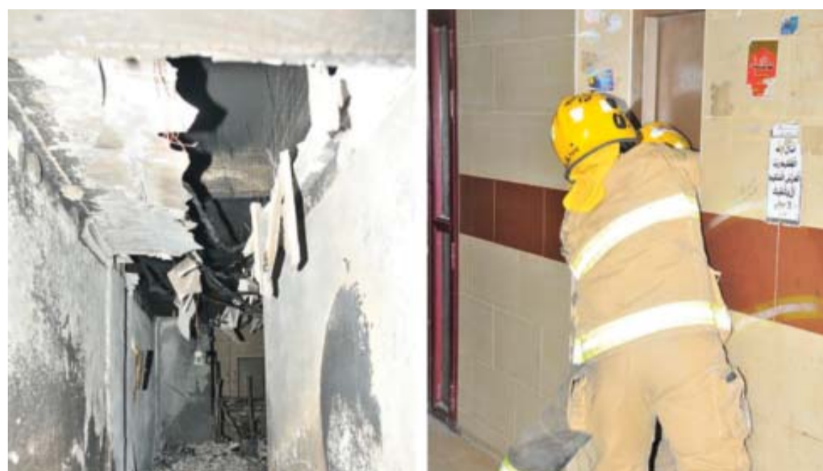
KUWAIT: Four children were killed in a fire in a sixth-floor flat in Farwaniya yesterday. Furniture, mattresses and other objects in the stairwell hindered firemen as they tried to reach the affected apartment, while residents of the building were evacuated. One fireman was injured. — By Hanan Al-Saadoun
