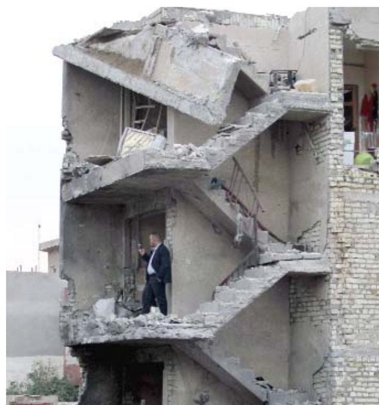
BAGHDAD: A Iraqi man checks a damaged building near the Al-Jawaher Mall in eastern Baghdad the day after a bomb attack yesterday. — AFP
