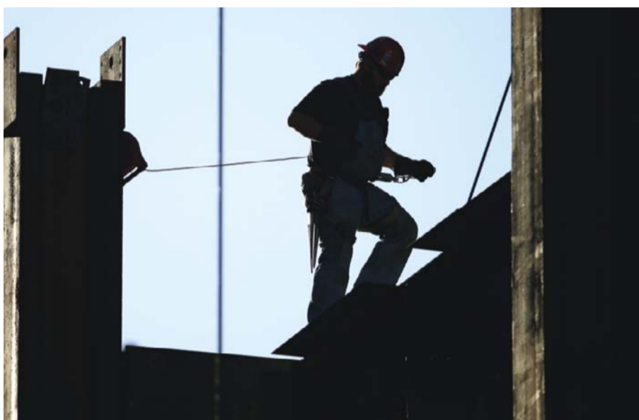
PHILADELPHIA: A worker works on the new Comcast Innovation and Technology Center under construction, in Philadelphia. The Commerce Department reports on US construction spending in November on Monday. —AP
