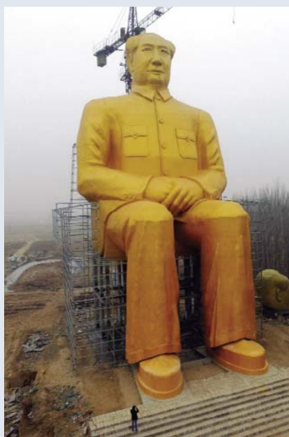
KAIFENG: Photo shows a huge statue of Chairman Mao Zedong under construction in Tongxu county in Kaifeng, central China's Henan province. — AFP
