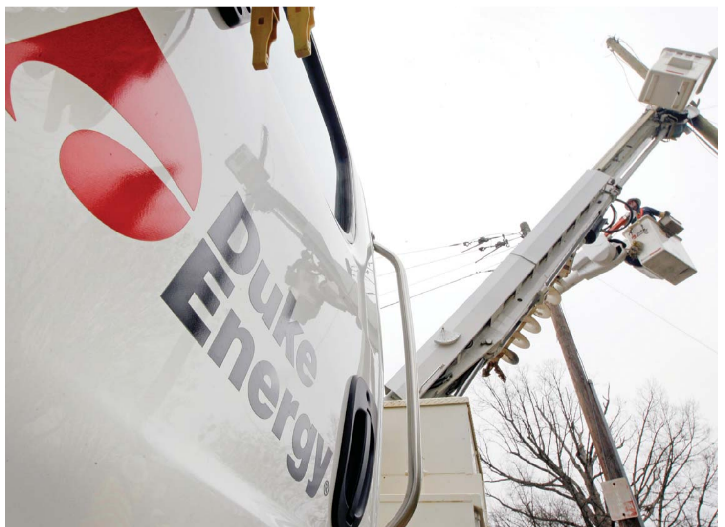
CHARLOTTE: Duke Energy employees work on power lines in Charlotte, NC. Utility stocks ended 2015 modestly lower. —AP
