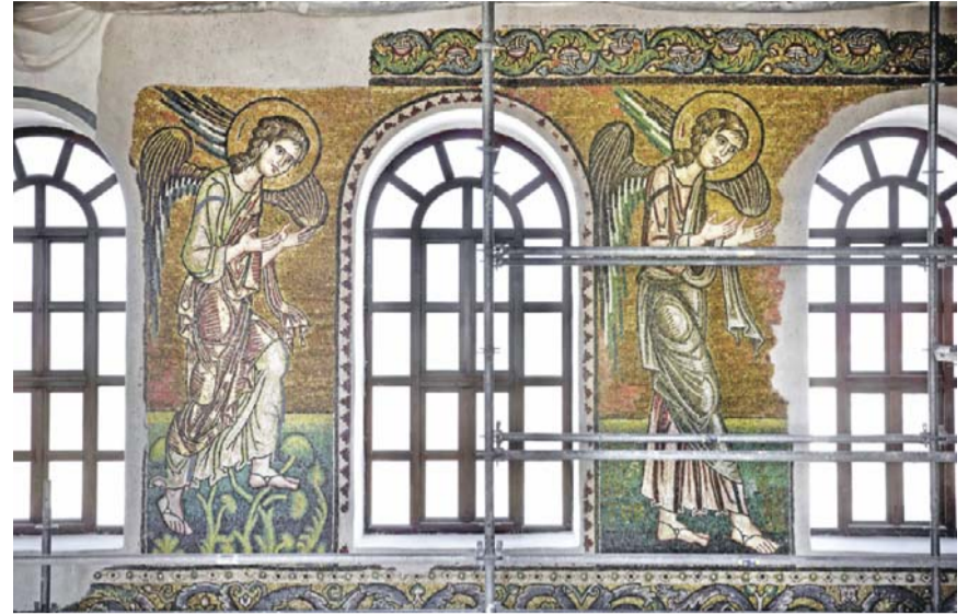
BETHLEHEM: Renovated mosaics and windows are the Church of the Nativity, in the West Bank city of Bethlehem.
