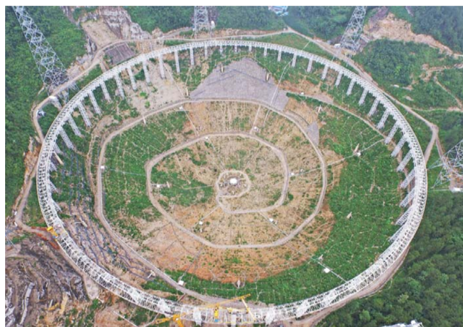
PINGTANG, China: This file picture taken on July 29, 2015 shows the 500-m Aperture Spherical Radio Telescope (FAST) under construction in southwest China's Guizhou province. — AFP
