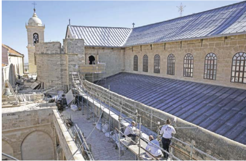
BETHLEHEM: Restoration experts work on the rooftop of the Church of the Nativity, in the West Bank city of Bethlehem. — AP photos
