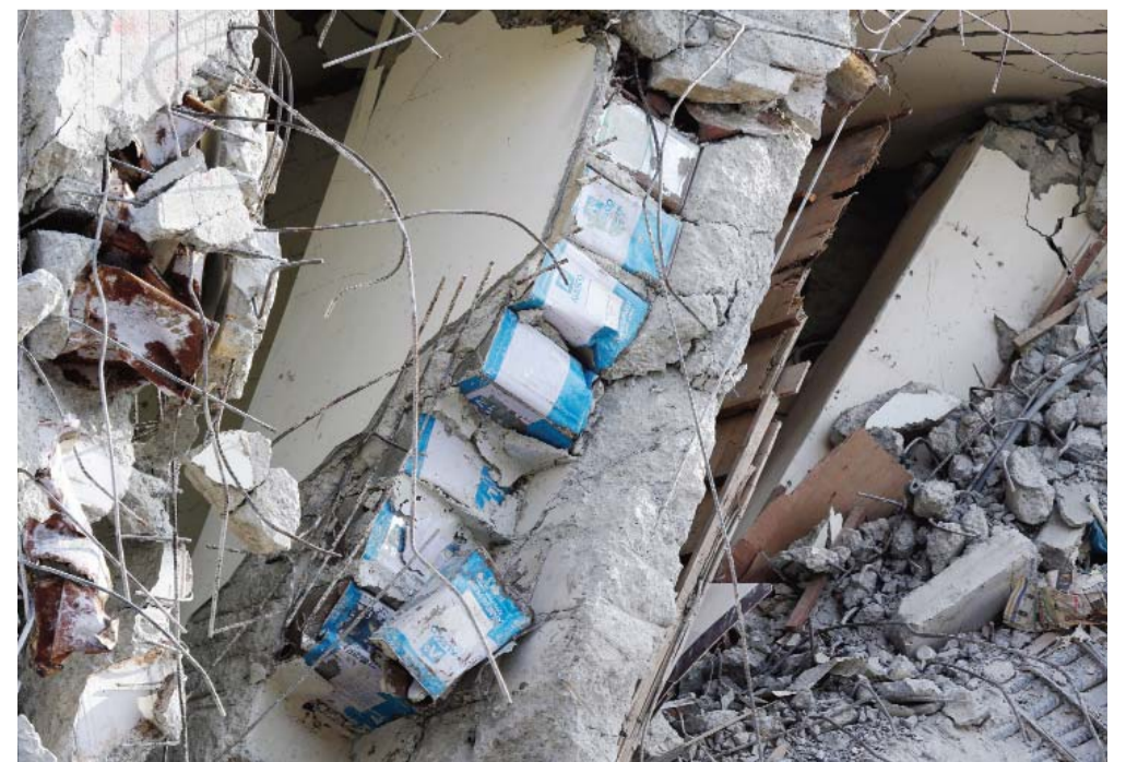
TAINAN: Tin cans are exposed in the cement structure of the collapsed building complex in Tainan, Taiwan. — AP
