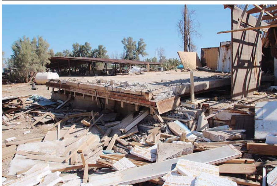
A collapsed ceiling at a building in a Wafra farm, which killed one worker yesterday.
