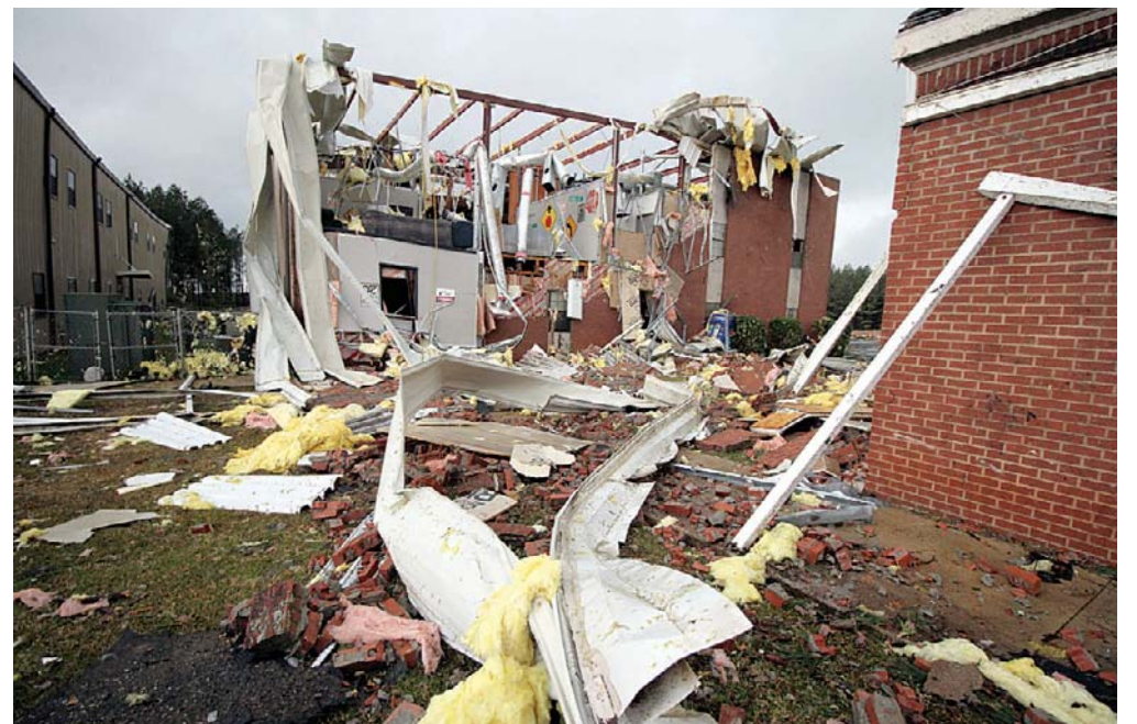
LAUDERDALE: Debris lies on the ground near First Baptist Church of Collinsville in Lauderdale County, Miss after it was severely damaged during a storm. —AP
