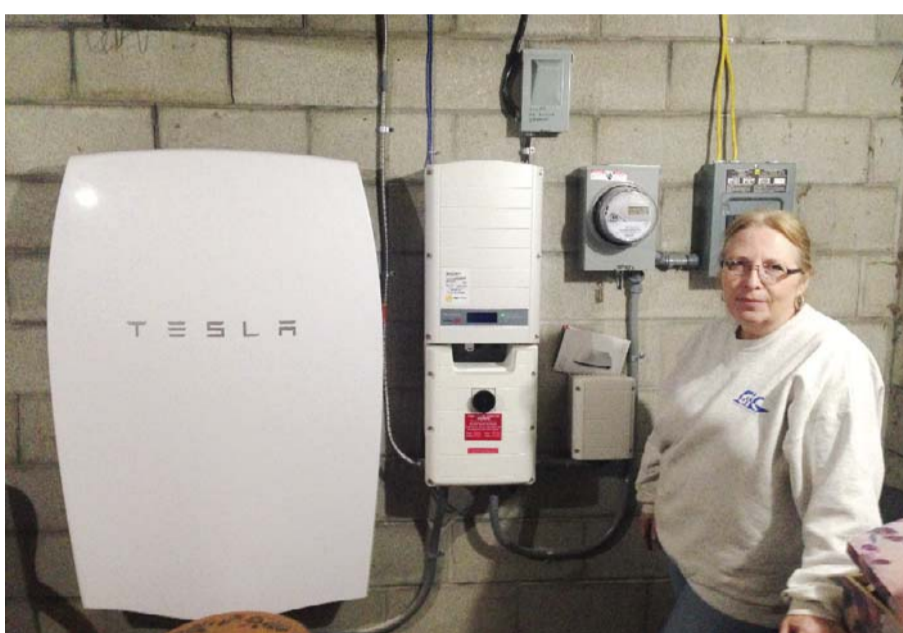
MIDDLETOWN SPRINGS: In this photo, Rhonda "Honey" Phillips poses next to a Tesla Powerwall battery and inverter connected to a solar panel array in her yard in Middletown Springs, Vermont. —AP
