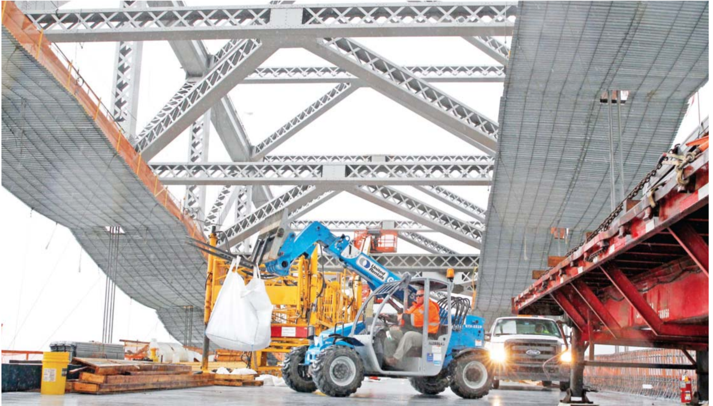
BAYONNE: In this Nov 15, 2016, file photo, a worker lifts materials as construction continues on the new roadway deck of the Bayonne Bridge in Bayonne, NJ. Even as they maneuver for a share of the $1 trillion in spending President-elect Donald Trump promised to rebuild America's roads, bridges and airports, lobbyists for transportation and utility industries are beginning to wonder whether Trump really meant what he said. — AP
