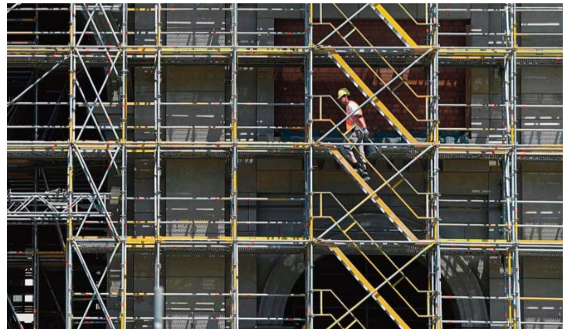
BERLIN: This file photo taken on June 6, 2016 shows a worker walking on a scaffolding at a construction site in Berlin. German businesses rounded off 2016 with a stronger-than-forecast increase in confidence, a closely-followed survey showed yesterday. —AFP
