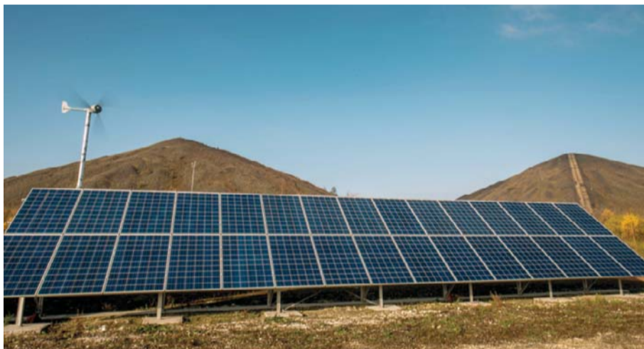
PAS-DE-CALAIS, France : A picture shows a wind turbine and solar panels installed at the Lumiwatt site, a site of research and testing on photovoltaic panels. — AFP
